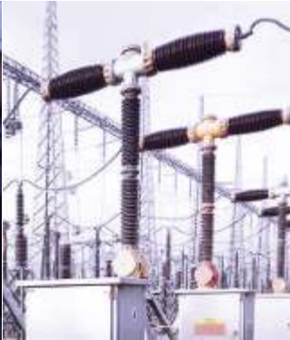
CORONA, PARTIAL DISCHARGE DETECTION
